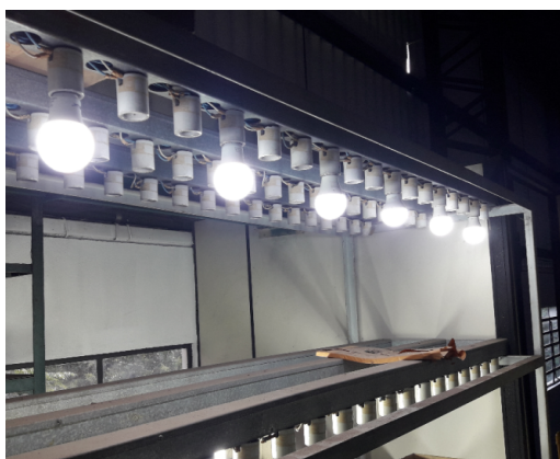
Figure 3: Rack with six light-emitting diode (LED) lamps left on for 24 hours/day.
